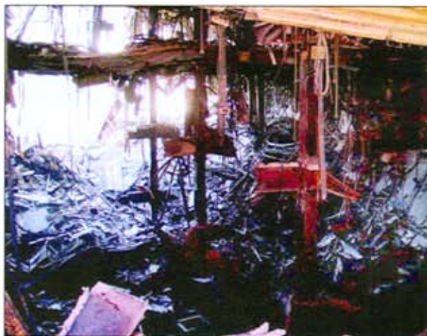
Figure 5: Internal collapsed areas in WTC 5.
