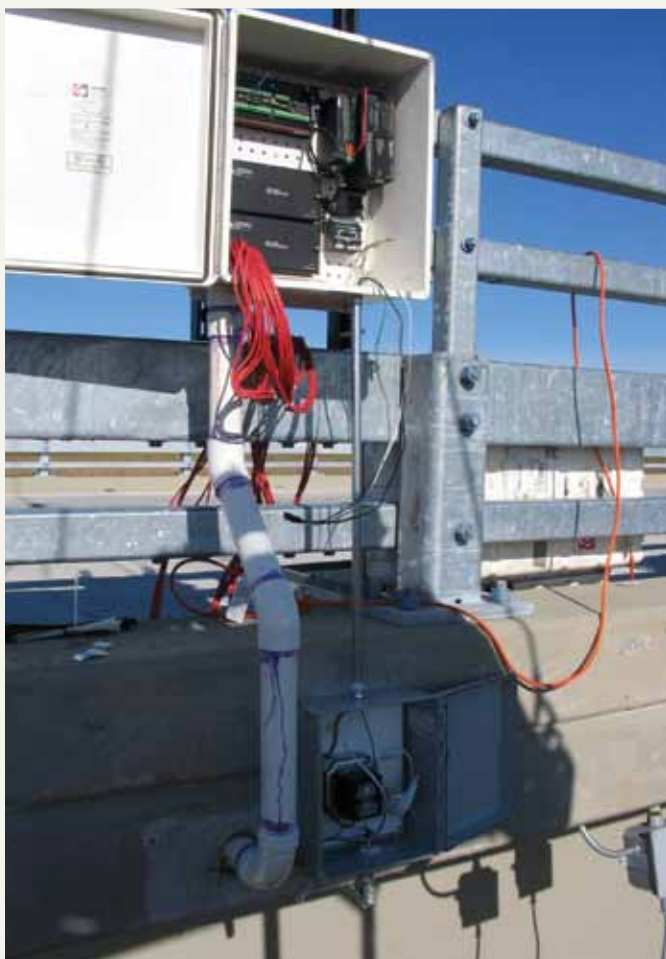
Figure 5. This automated data acquisition system was installed on the south guardrail of span 43.
