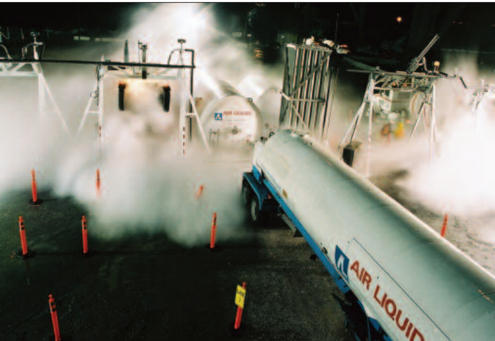
Top: Liquid nitrogen was injected into the ready mix trucks at this lancing station, shown here one with lance extended and one retracted. Bottom: Precooling concrete with liquid nitrogen generates a white fog, as water vapor in the air is also cooled below the dew point. Gaseous nitrogen is colorless, tasteless, and odorless.
