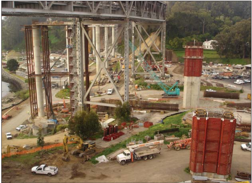
CTLGroup worked with a majority of the contractors involved in the project to develop their thermal-control plans and aided in the selection of the most appropriate and cost-effective means of thermal control.
